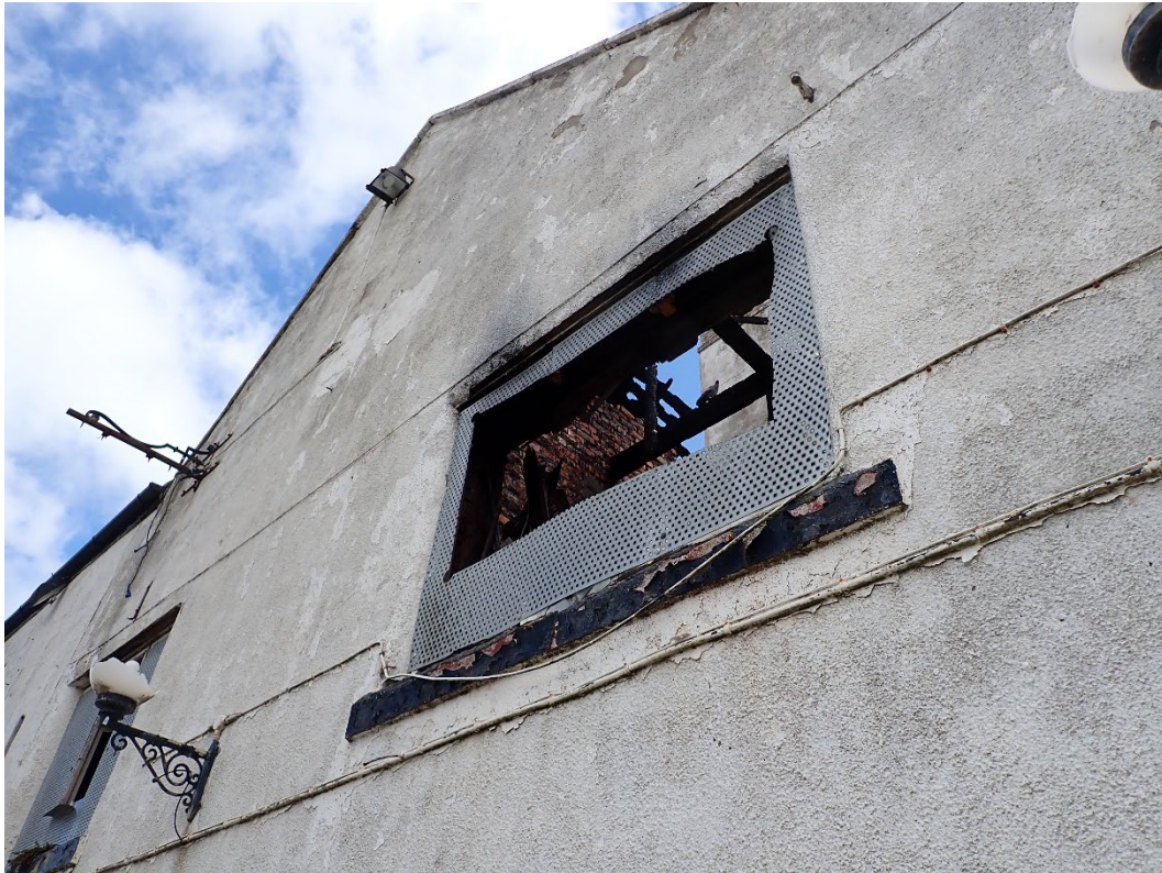
Photo 7: Internal walls and roof trusses are visible through the windows, looking north-east
