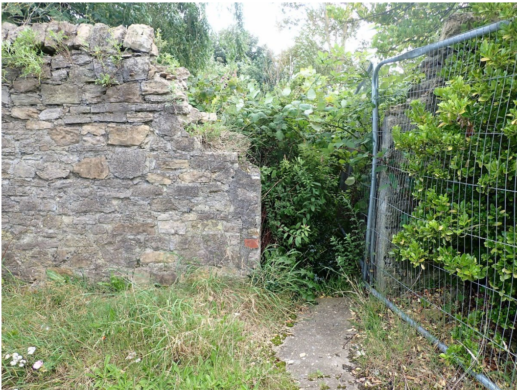
Photo 10: The former garden to the south is now an impenetrable mass of shrubs and plants, looking south
