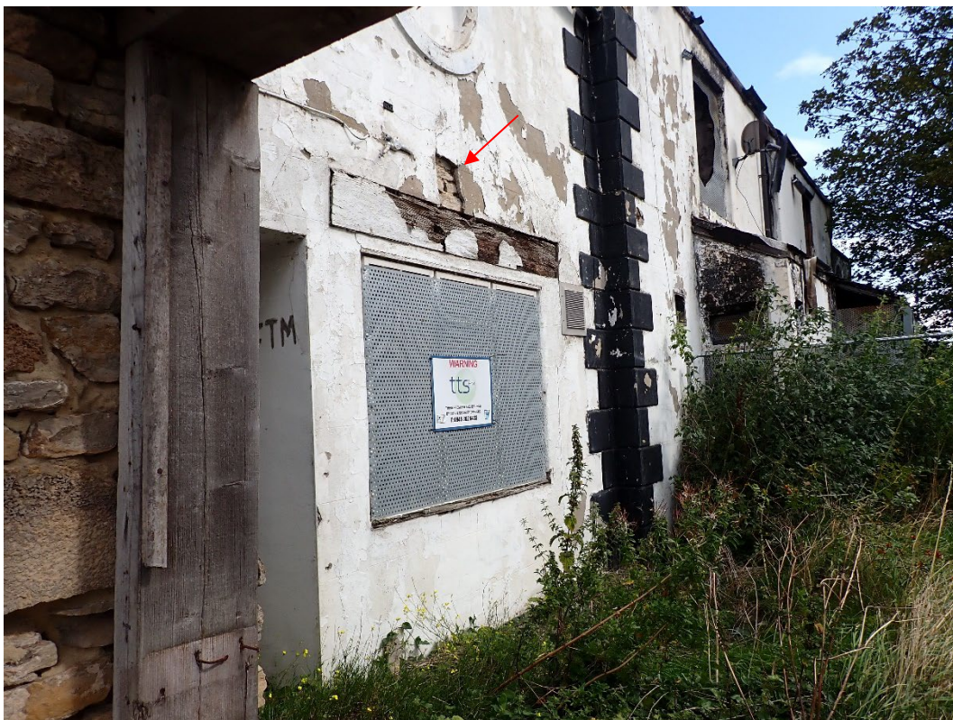
Photo 8: The render is coming away on the southern elevation of the building, looking north-east
