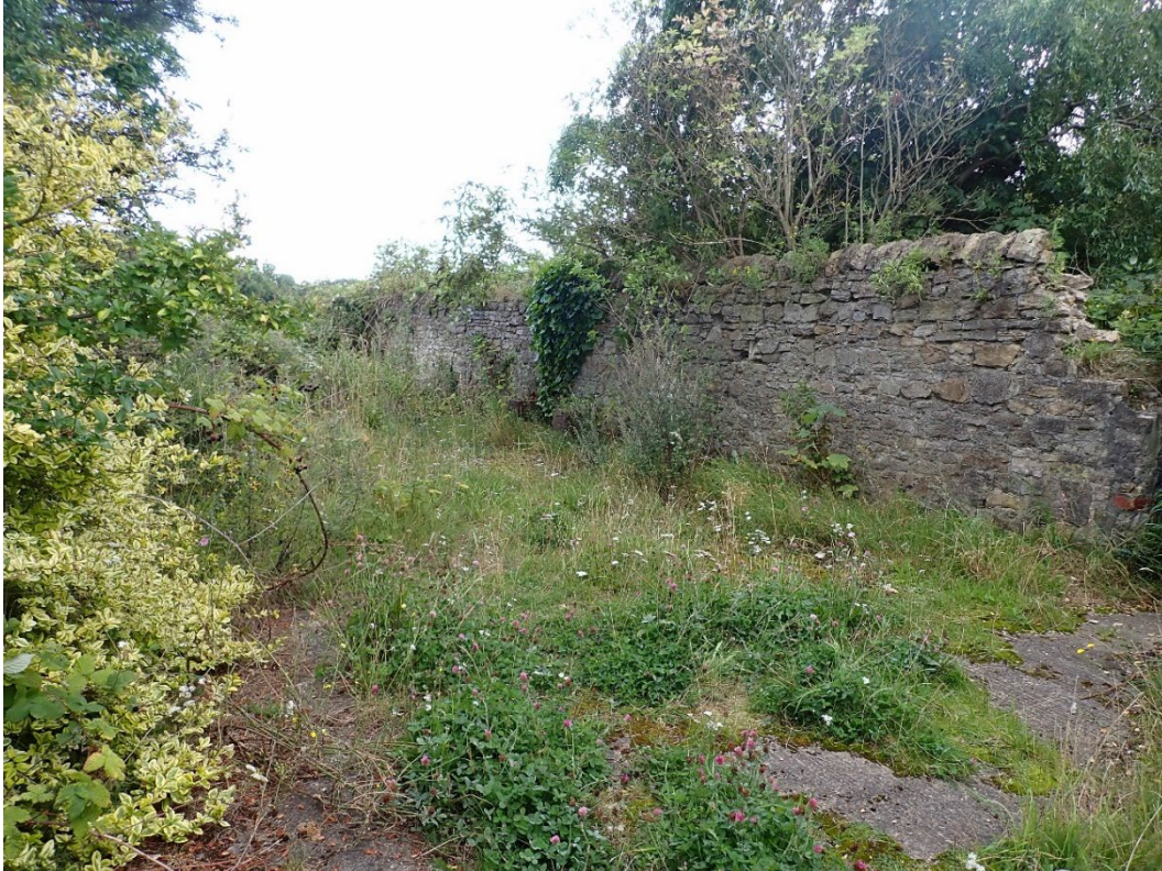
Photo 9: The stone wall to the east of the burnt building, looking south-east
