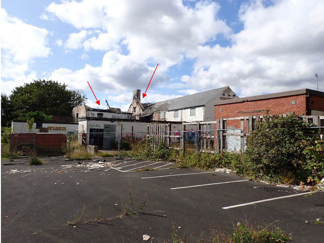
Photo 5: The derelict pub is fenced off. The oldest part of the building is partially burnt down (highlighted), looking south-west
