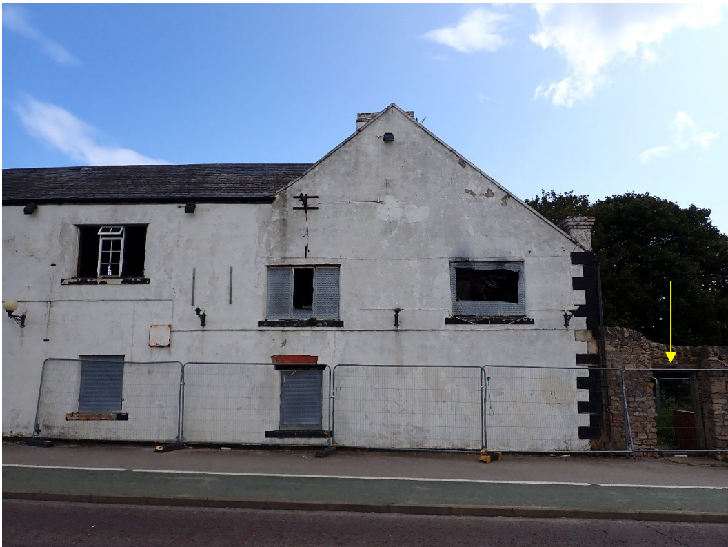
Photo 6: In some cases, the boarding on the windows has been broken or removed. The entrance into the southern area can be seen on the right, looking east
